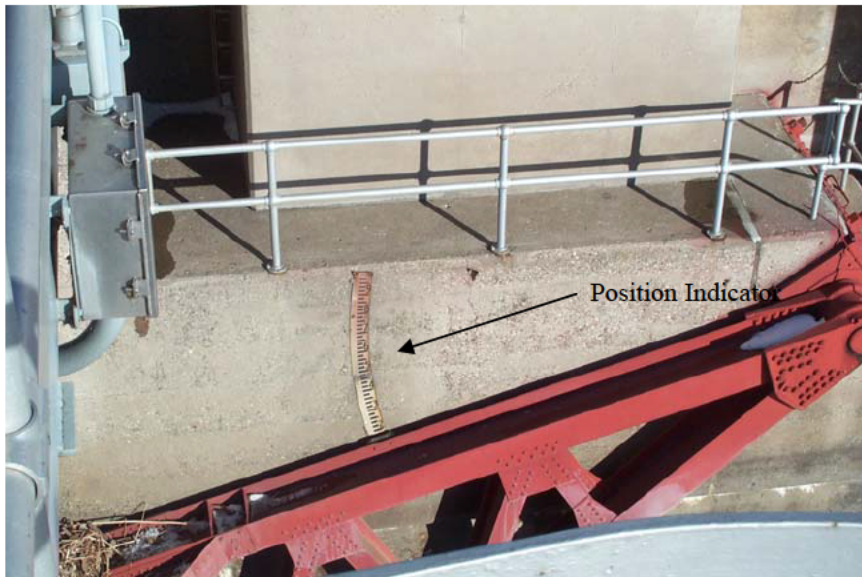
Figure 2-4. Tainter Gate Position Indicator
