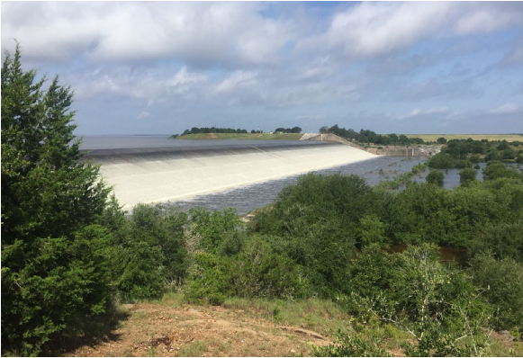
Figure 4-7. Somerville Dam Overtopped
