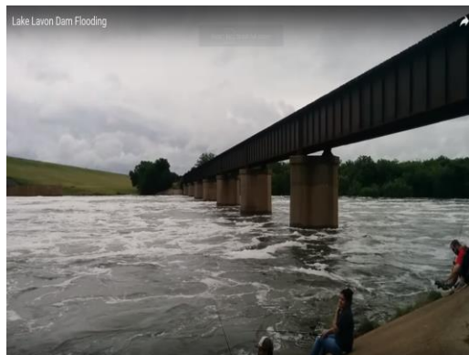
Figure 4-3. 2015 Flood - High Water Level at Price's Creek Bridge
