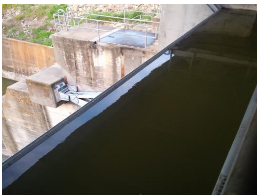
Figure 4-4. 2015 Flood – Flooded Dam Bridge
