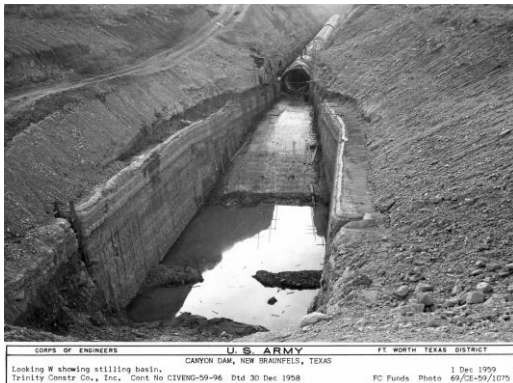
Figure 3-1. Outlet Works Stilling Basin, 30 December 1958
