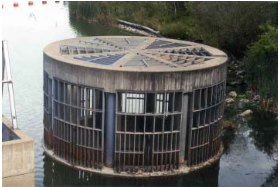
Figure 2-2. Morning Glory Inlet and Trash Rack
