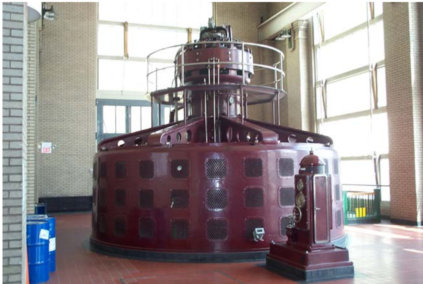
Figure 2-4. Westinghouse Generator Unit No. 1
