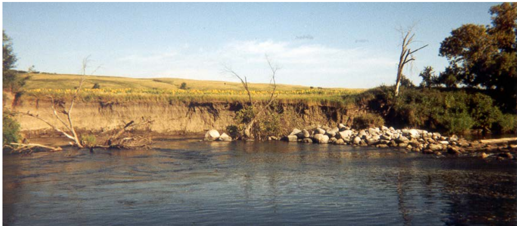
Figure 3-1. Scour of the Tailwater Gaging Location
