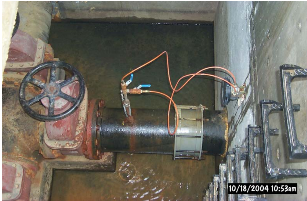
Figure 7-1. USFWS Siphon Well and Water Meter
