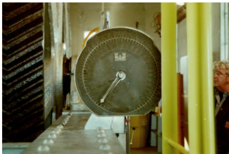
Figure 2-3. Alternate Roller Gate Position Indicator
