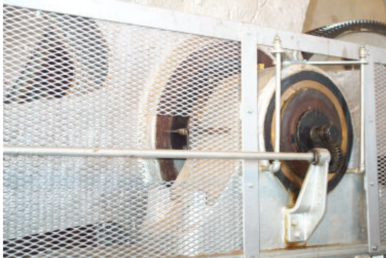
Figure 2-2. Roller Gate Position Indicator
