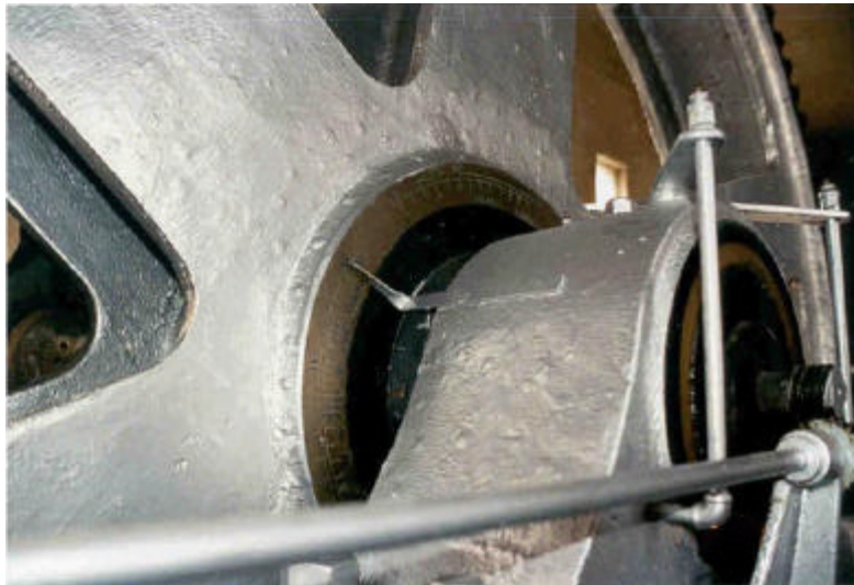
Figure 2-2. Roller Gate Position Indicator
