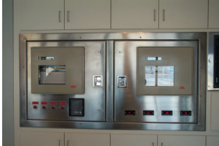
Figure 5-3. Stevens PAV-C Pool and Tailwater Elevation Recorders
