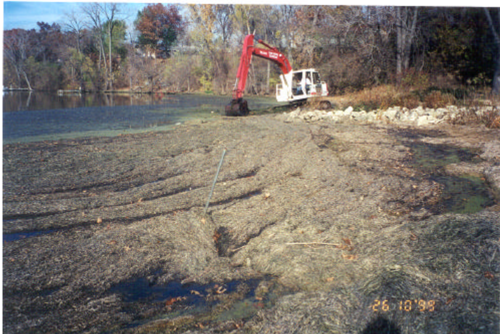
Figure 3-1. French Lake Aeration Culvert.
