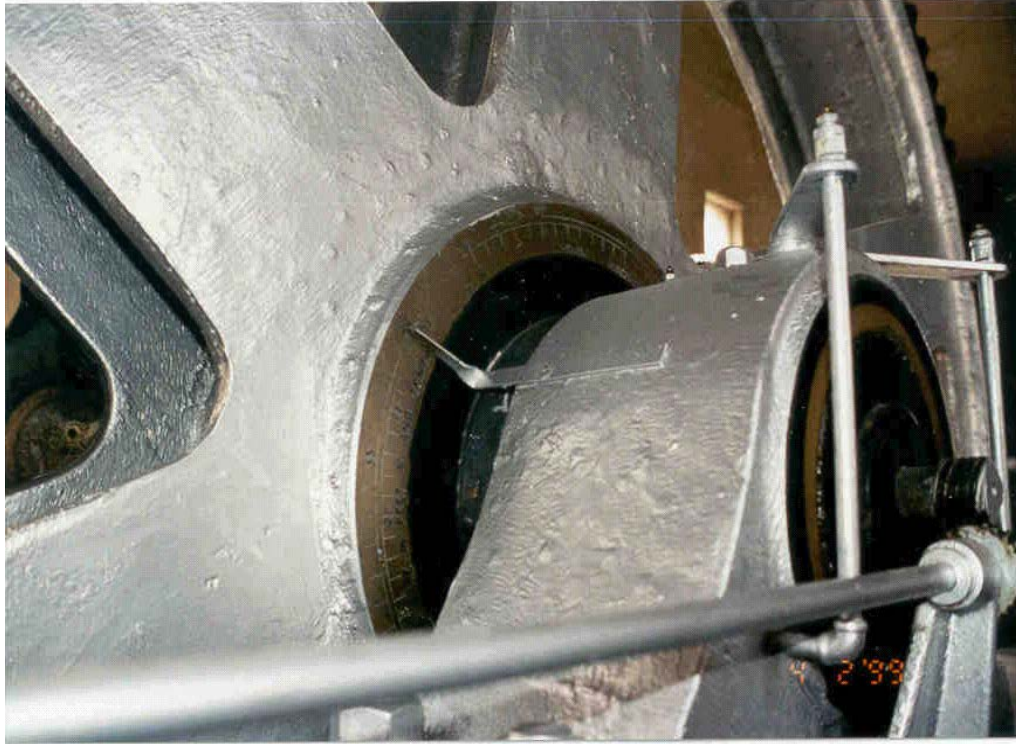
Figure 2-2. Roller Gate Position Indicator
