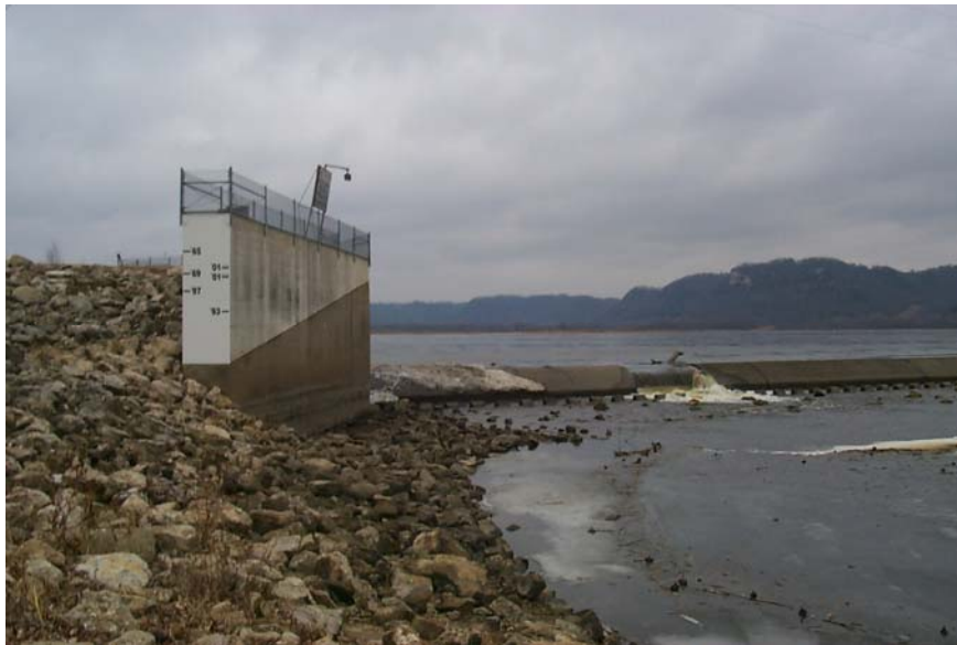
Figure 2-5. Concrete Spillway with Notch.
