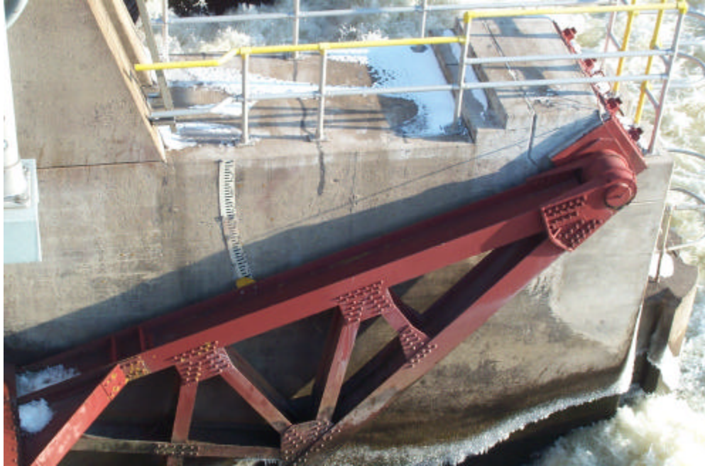
Figure 2-3. Tainter Gate Position Indicator
